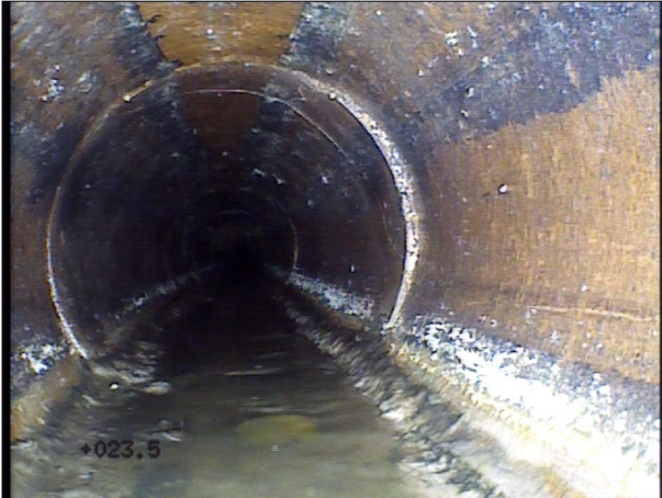
Photo: 36a, Tape No.: 7 23.5m, Circumferential Crack at joint, from 11 to 04 o'clock
