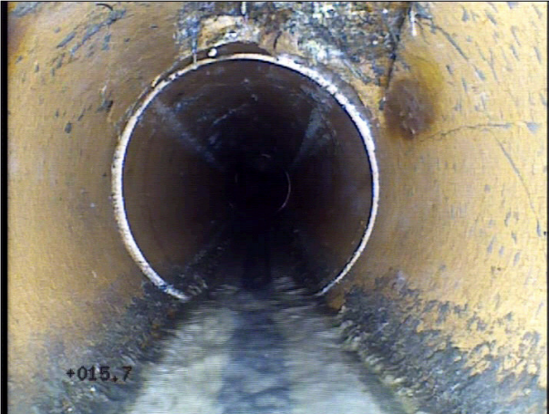
Photo: 14a, Tape No.: 3 15.7m, Hole in sewer from 12 to 02 o'clock
