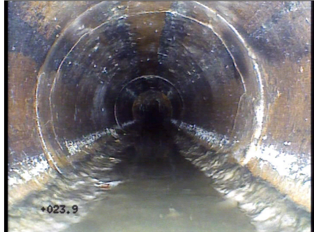
Photo: 37a, Tape No.: 7 23.9m, Circumferential Crack at joint, from 07 to 04 o'clock
